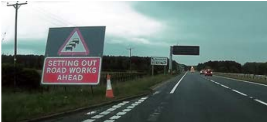
Figure A.11 Roadside sign during the enhanced mobile carriageway closure trials with vehicle downstream
